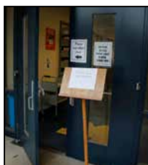
The ARC door that is scheduled to be fixed. Photo by Emma Pindell '13
